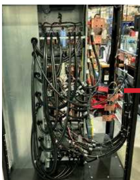
Cabinet with cables
