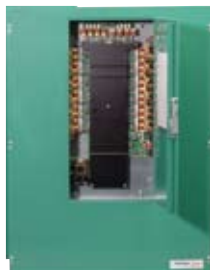
Lighting Control Panel
